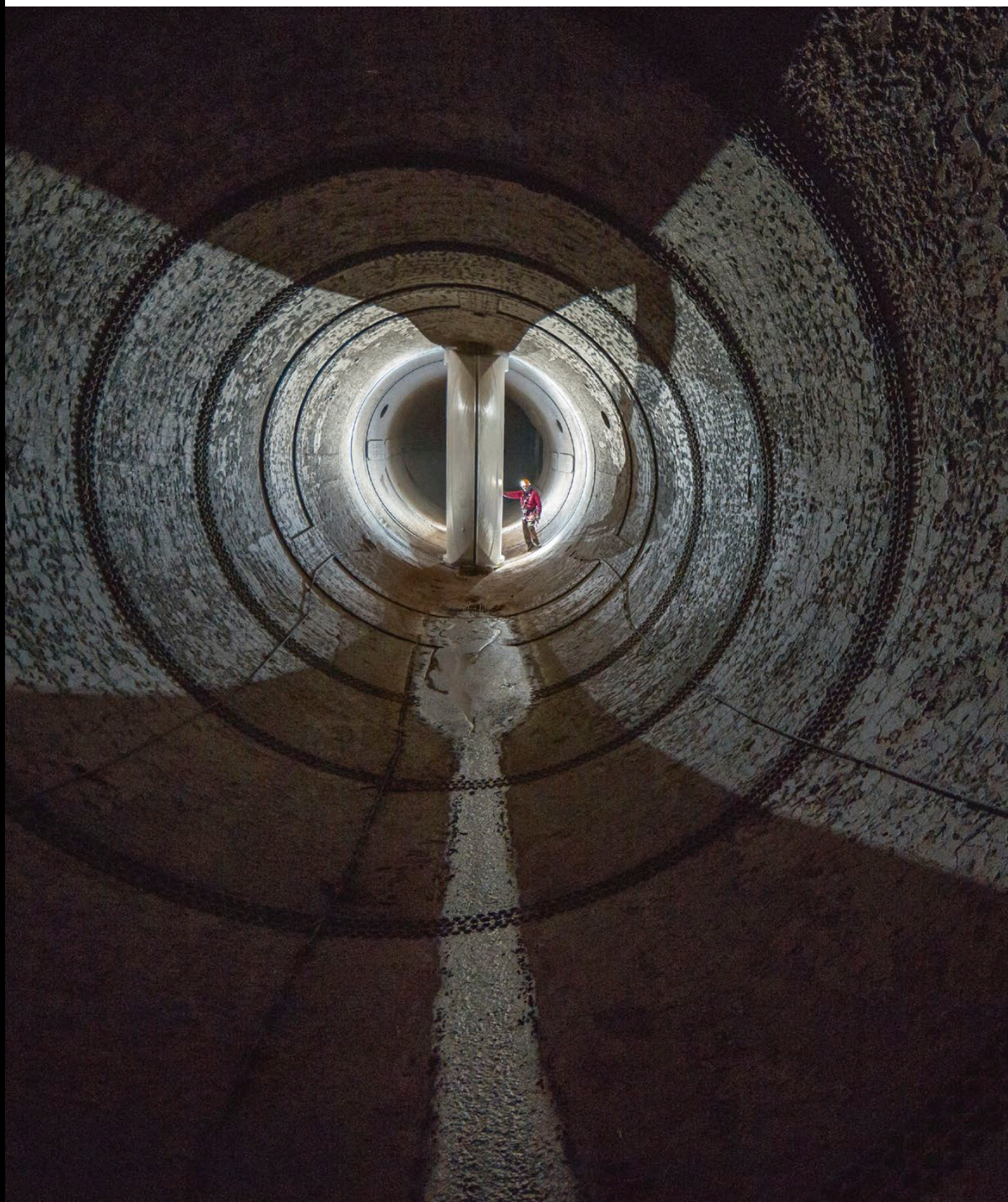
Inspection of the penstock and circular valve deep inside a dam. © Petzl / Lafouche / Systeme Corde
