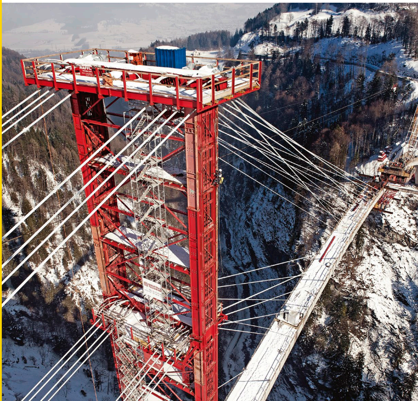
Construction of the LGB Lehergerüstbau in Taminaabrücke, Pfäfers, Switzerland. © Ing. Bernhard Roggen
