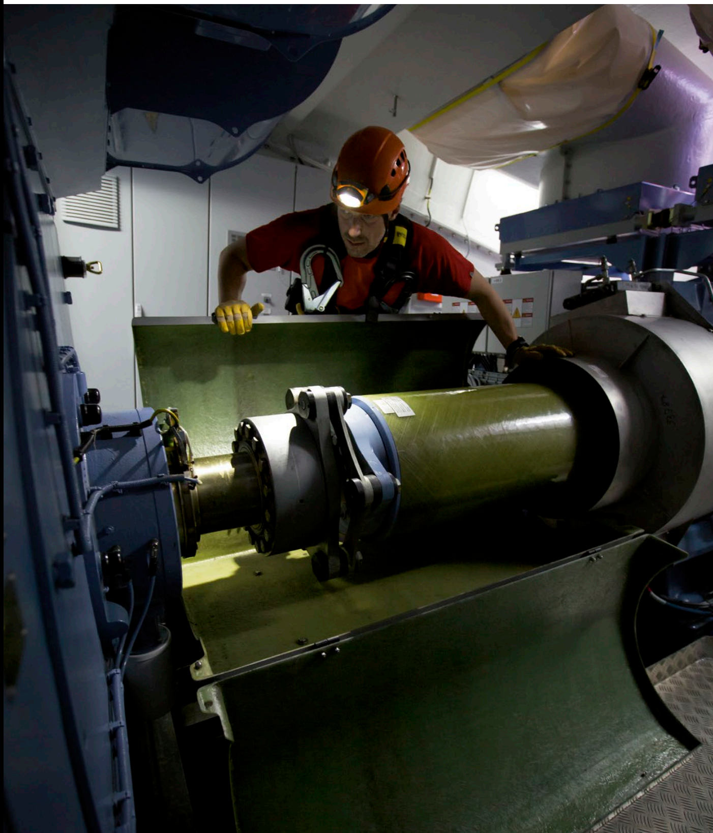
Maintenance operations in the nacelle of a wind turbine in Deining, Germany. © Petzl / Lafouche / Max Bögl
