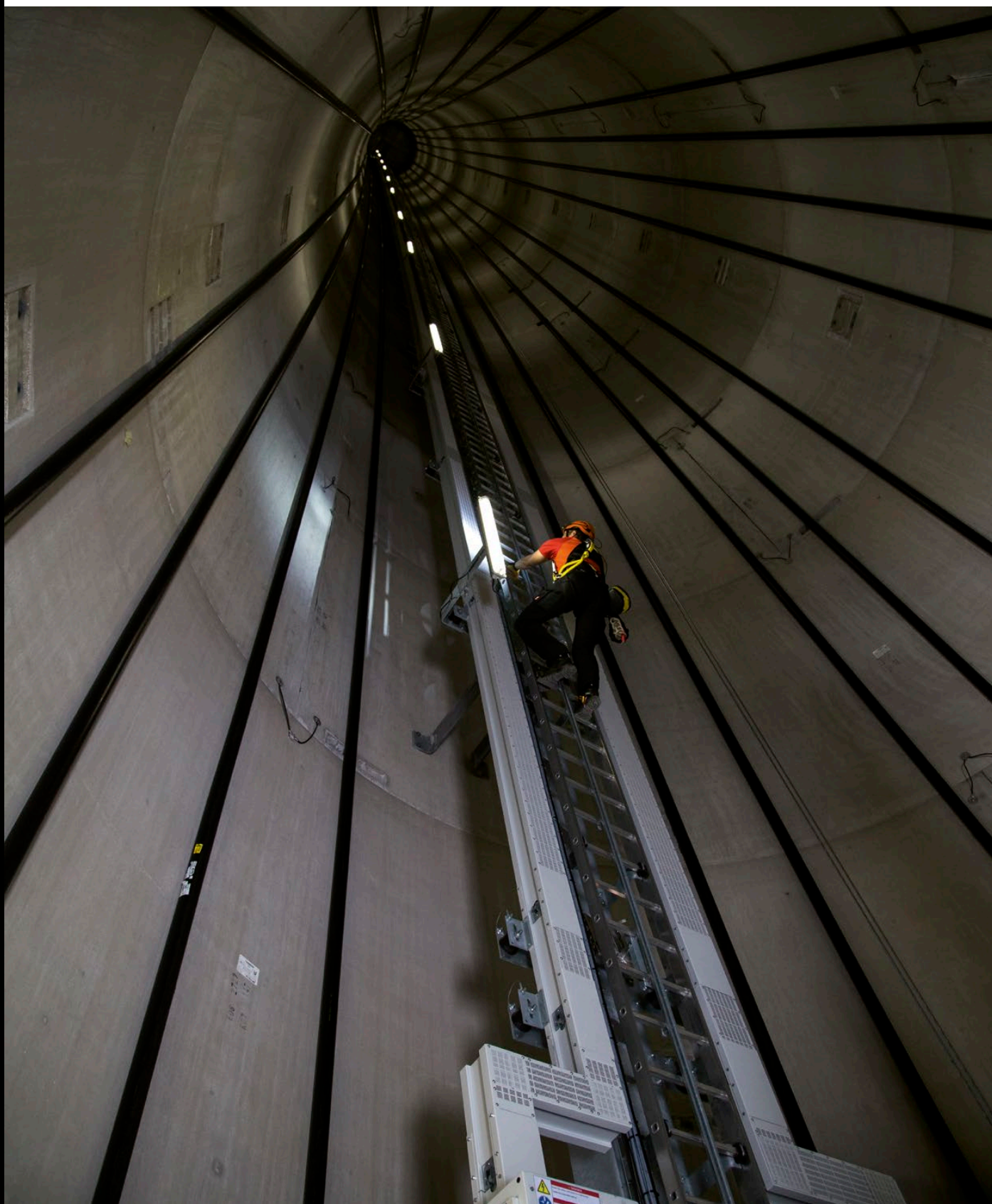
Maintenance operations in the shaft of a wind turbine in Deining, Germany. © Petzl / Lafouche / Max Bögl
