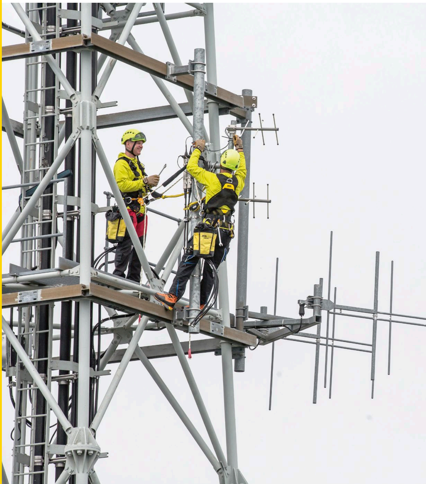
Antenna maintenance work on the Monte San Salvatore tower in Lugano, Switzerland. © Petzl / Lafouche / Swisscom Broadcast / Etavis
