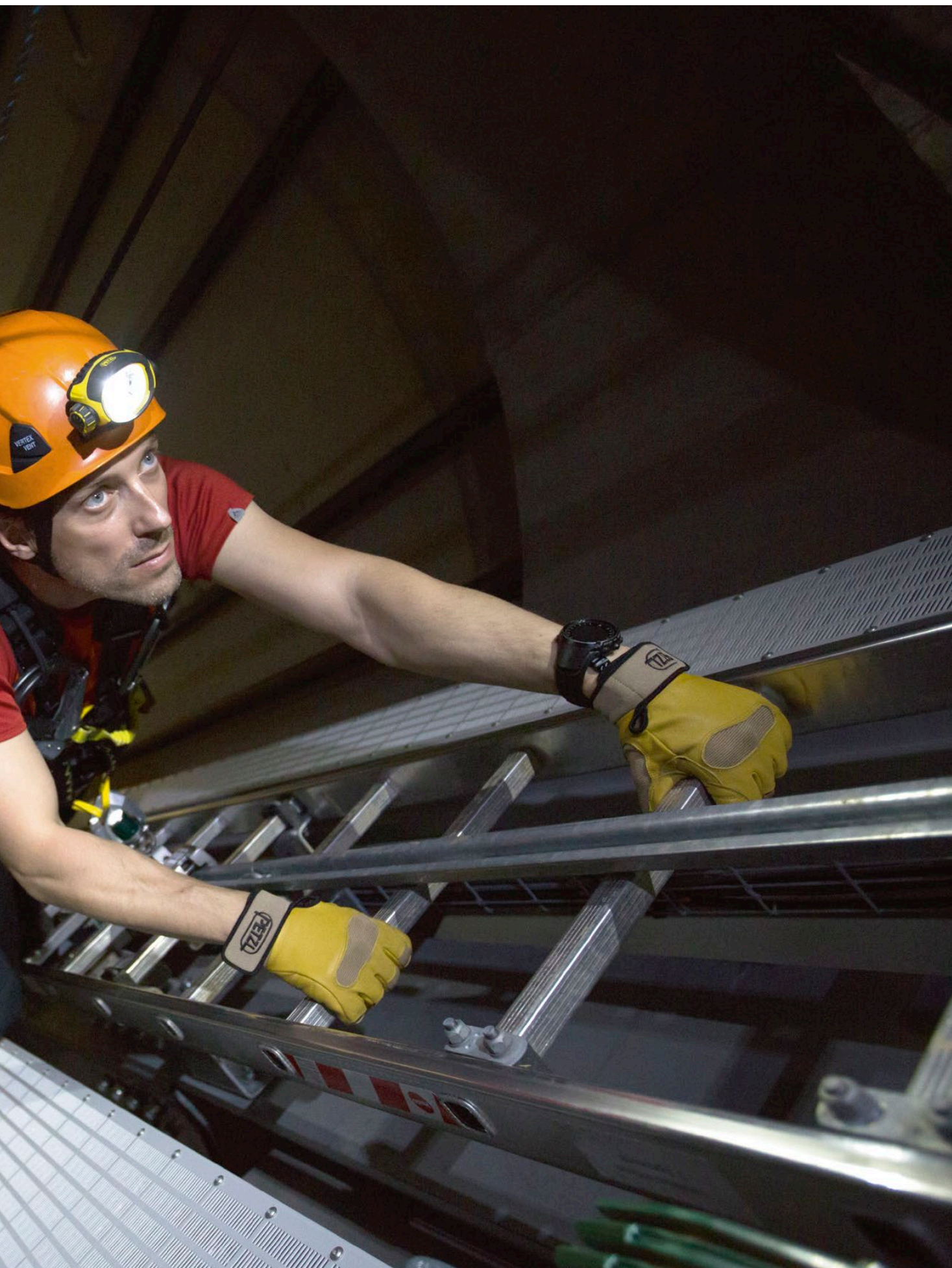
Maintenance operations in the shaft of a wind turbine in Deining, Germany. © Petzl / Lafouche / Max Bögl
